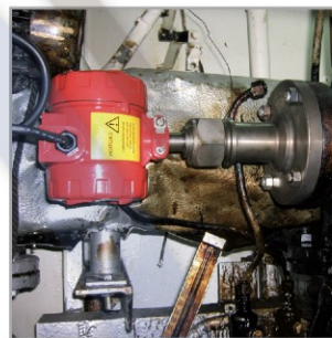
After - VISCOMASTER retrofit
